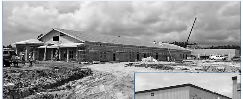
The construction for the new school building should be complete in early 2014.
